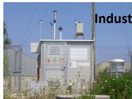
AQ monitoring station by ARPA-PUGLIA, IT
