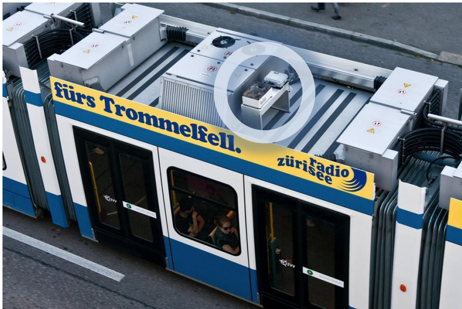
Sensor nodes are installed on top of streetcars
