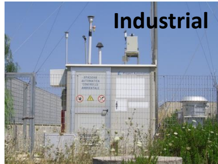
AQ monitoring station by ARPA-PUGLIA, IT
