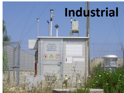
AQ monitoring station by ARPA-PUGLIA, IT
