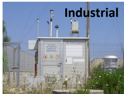
AQ monitoring station by ARPA-PUGLIA, IT
