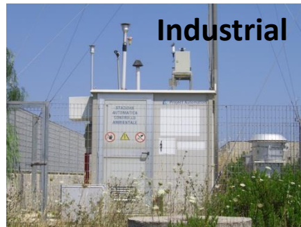
AQ monitoring station by ARPA-PUGLIA, IT
