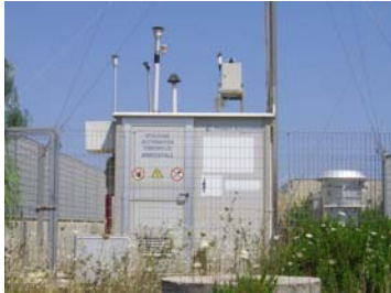
Figure 4. Air Quality Monitoring Station of ARPA-Puglia, Environmental Protection Regional Agency (Bari, Italy).
